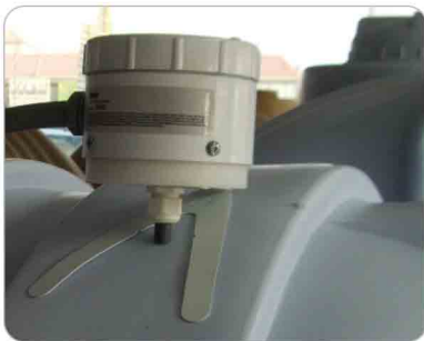
Mounting at horizontal polyethylene water tank using tripod hook.
