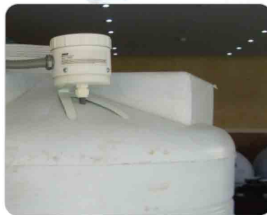
Mounting at vertical polyethylene water tank using tripod hook.
