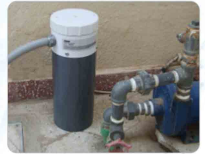
Direct mounting at concrete ground reservoir with \varnothing 152\text{mm} PVC sleeve.
