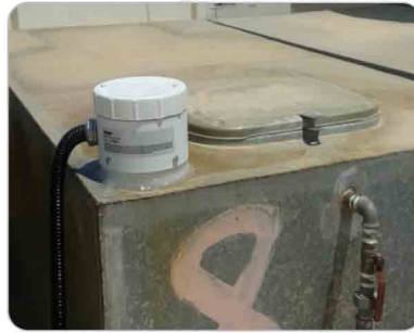
Direct mounting at steel water tank.
