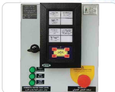
Alarm Annunciator Panel.
