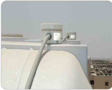
Direct mounting at flat head polyethylene tank.
